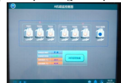
Intelligent Automation Interface of Cooling Towers at NKY Pharmaceuticals
