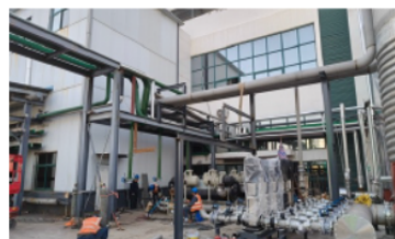
Implementation of Energy-saving Upgrade for the Chiller System in Workshop 102 by NKY Pharmaceuticals
